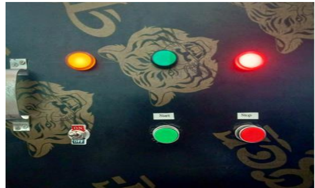
Figure 10 (a). Control Panel Result for Stop Condition
